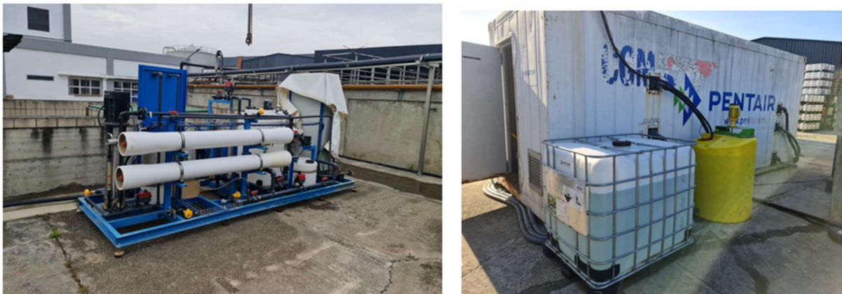
Figure 57. Pictures of RO (left) and NF (right) pilot plants used for the water reclamation case in CS5.
