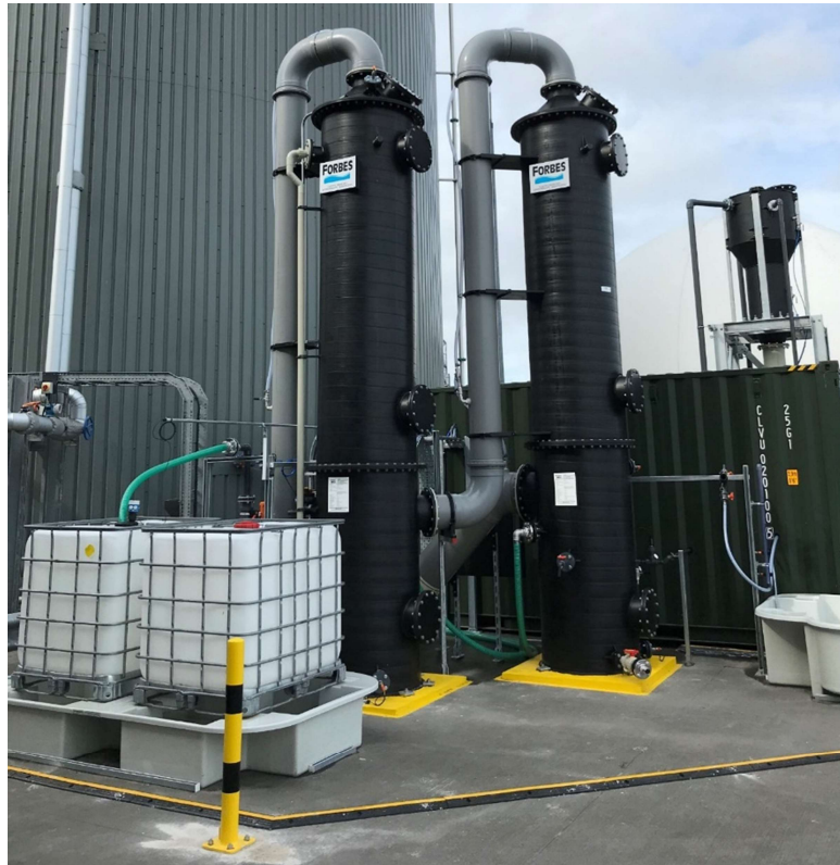
Figure 96. Ammonia stripping/scrubbing unit.
