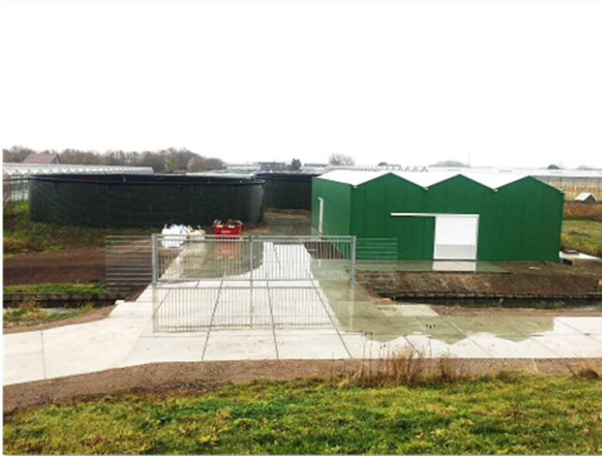
Figure 20. Treatment plant De Vlot.
