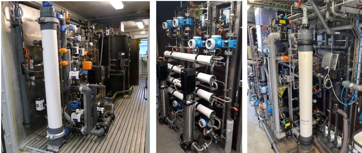
Figure 116. Pilot A - left: conventional ultrafiltration module; Pilot B - middle: reverse osmosis units and right: novel UF/NF module.
