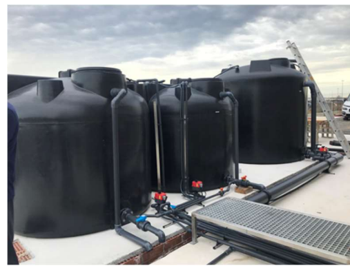
(b) Storage tanks
