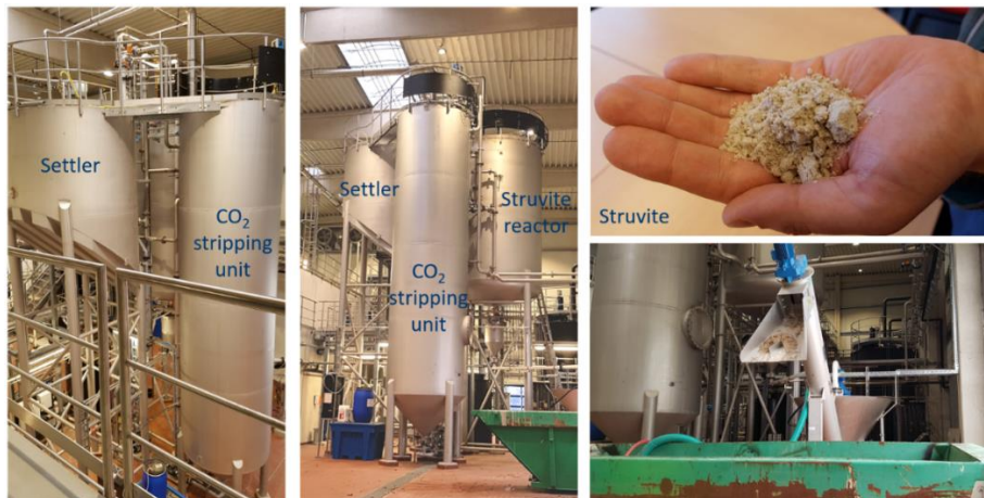
Figure 59 Pictures of the struvite production unit consisting of a CO2 stripping unit, a struvite reactor, a settler and a container to collect the harvested struvite crystals (NuReSys process).
