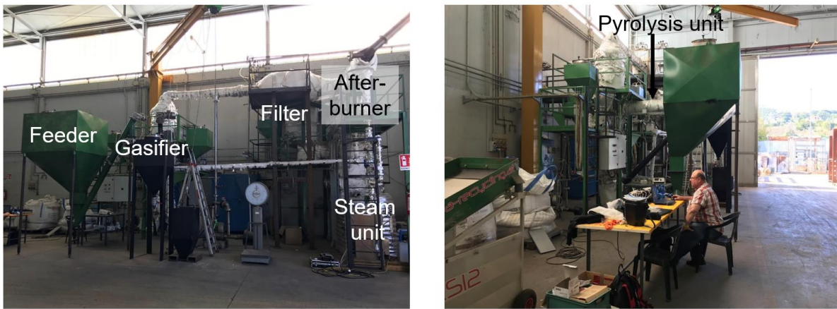
Figure 66 Front and side view of the pilot unit (picture owner: CTU)
