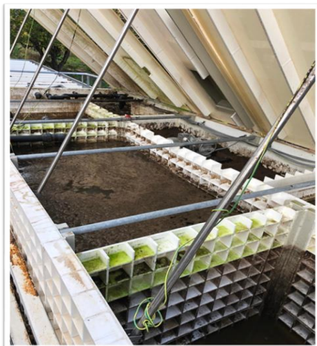
Figure 17. Various tanks of the treatment processes in the SM unit.
