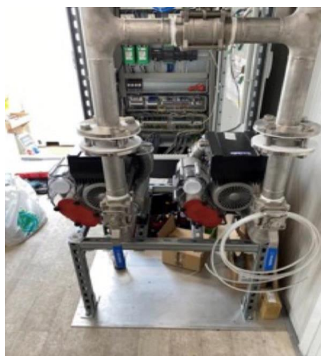
Figure 18. View of the interior of the container of the local control room.
