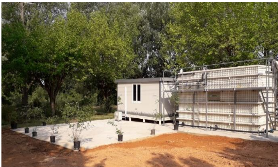
Figure 16. Overview of the sewer mining unit and the control room installed in the nursery.
