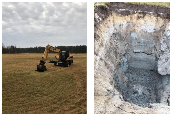
Figure 118. With the aim to visualize the ground water flocculation, a larger hole was dug in the same area where the larger borehole and its surrounding observation holes were drilled.
