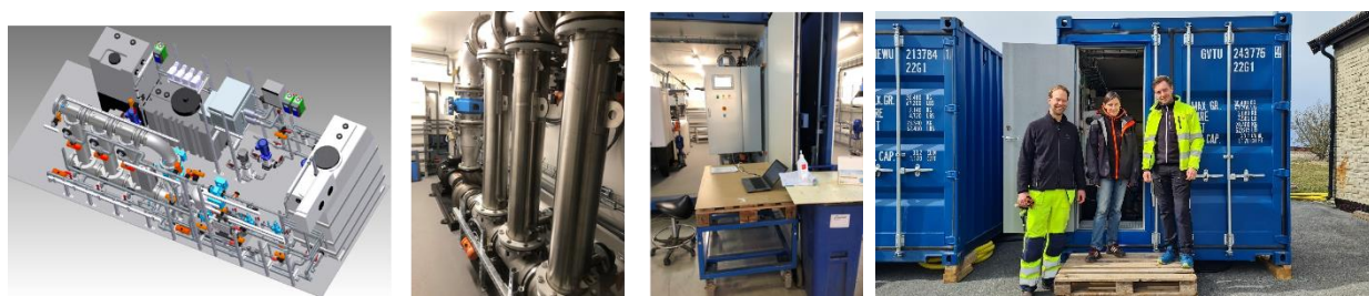
Figure 54. The containers for the ultrafiltration and reverse osmosis for direct reuse of water from sewage in Burgsvik, Storsudret.
