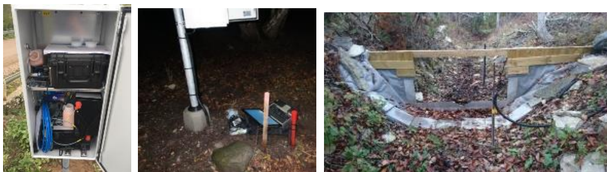
Figure 2. Images of the sensors for measuring surface levels and water flow for control of the automatic floodgates used in NextGen project. Left: One of the data collection boxes for receiving and sending the data to the Steven connect data platform, Middle: Calibration of a sensor in place, Right: a flow rate measuring control board with two sensors, one before the board and one after. From those data, the flow rate can be predicted.
